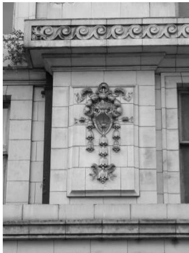
One of the many faience details that would be lost as part of the demolition scheme
