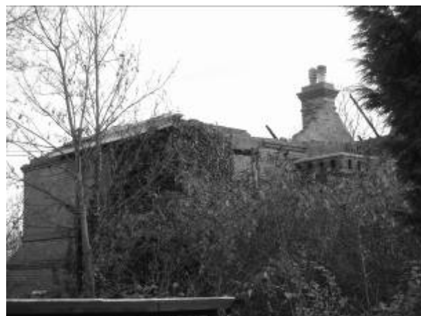
121 Ness Road – roofless and overgrown – a classic SAVE picture from over a fence and behind a tree
